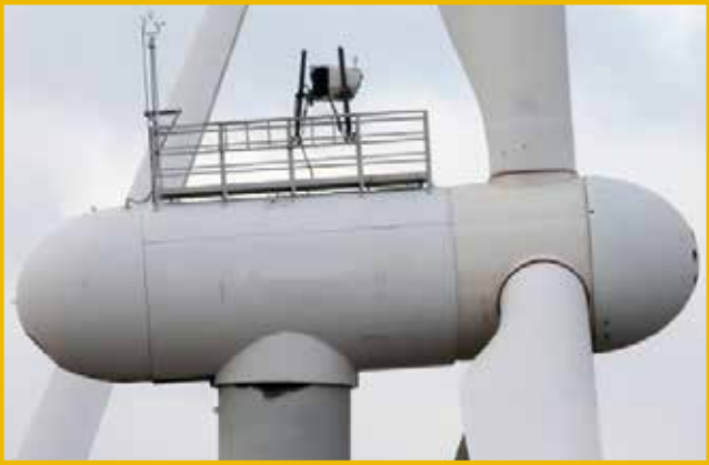
Wind turbine control
