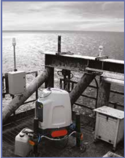
Forewind offshore platform
